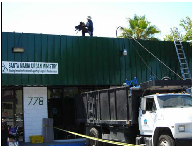
A worker from Shelton Roofers helps remove the old roof at Santa Maria.
